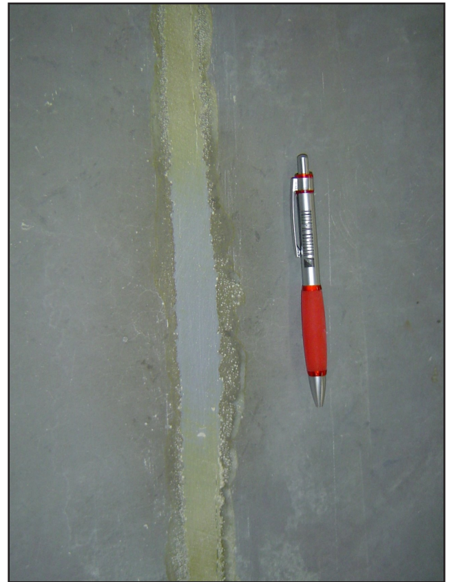
Photo above shows yellowing of the gray joint filler caused by the lighting system. The center of the joint was lightly sanded to show original filler color.
