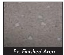
Ex. Filled Defect
