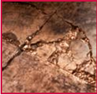
SLAB CORNER BREAKS
